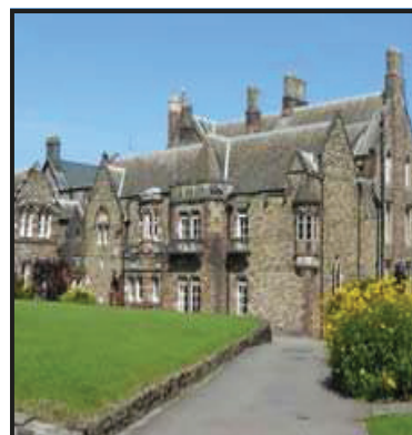
The 19th Century building is always in need of repair and upgrade.
